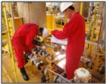
Pressure System Inspection
