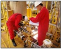
Pressure System Inspection
