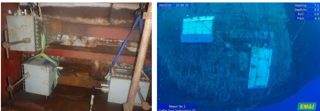
Internal ODIN winch boxes and external ODIN cofferdams
